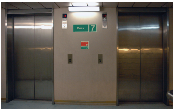
6434C (In case of fire do not use lift)
